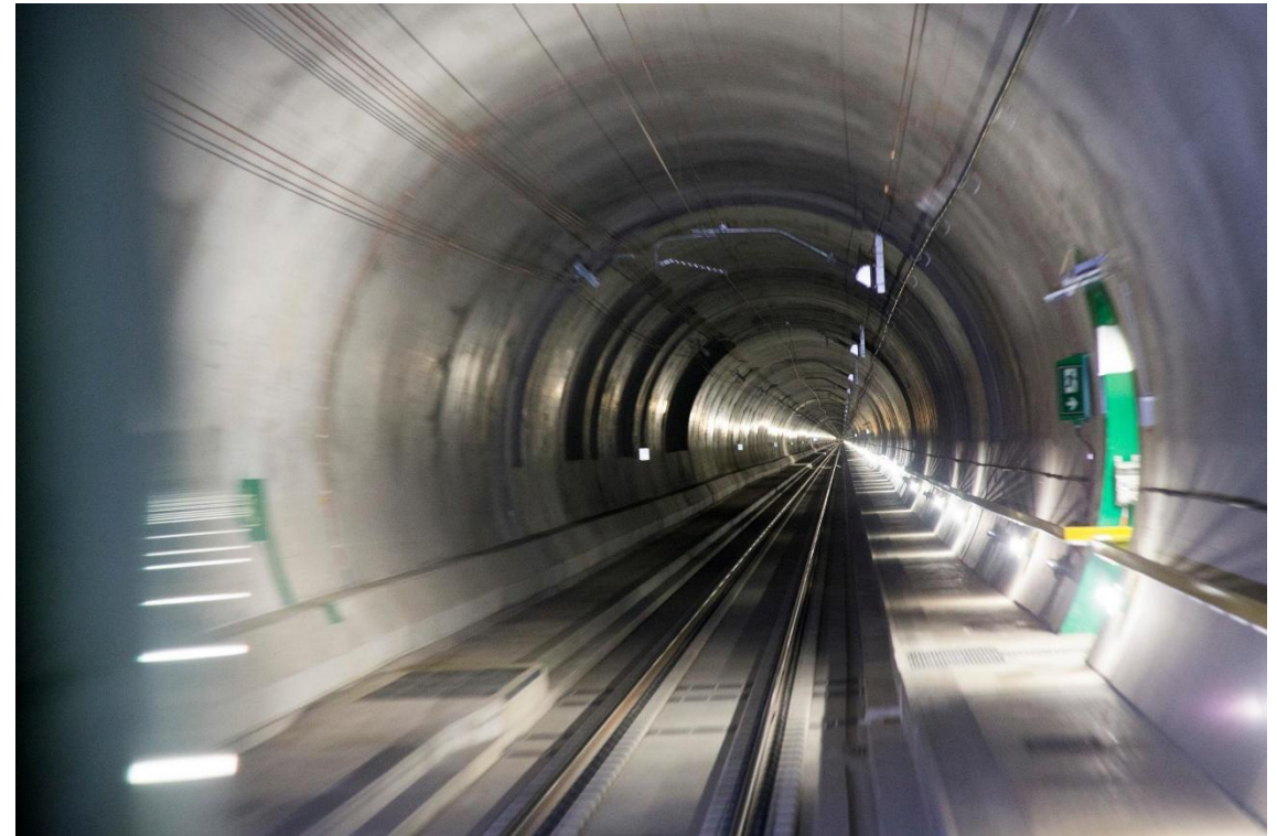
A modern tunnel consists of many electronic systems and a main challenge is the maintenance and renewal of this short-lived assets.
