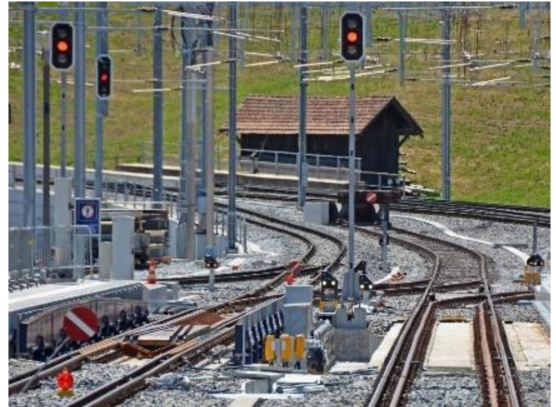
gauge-changing facility metre gauge – standard gauge Zweisimmen
